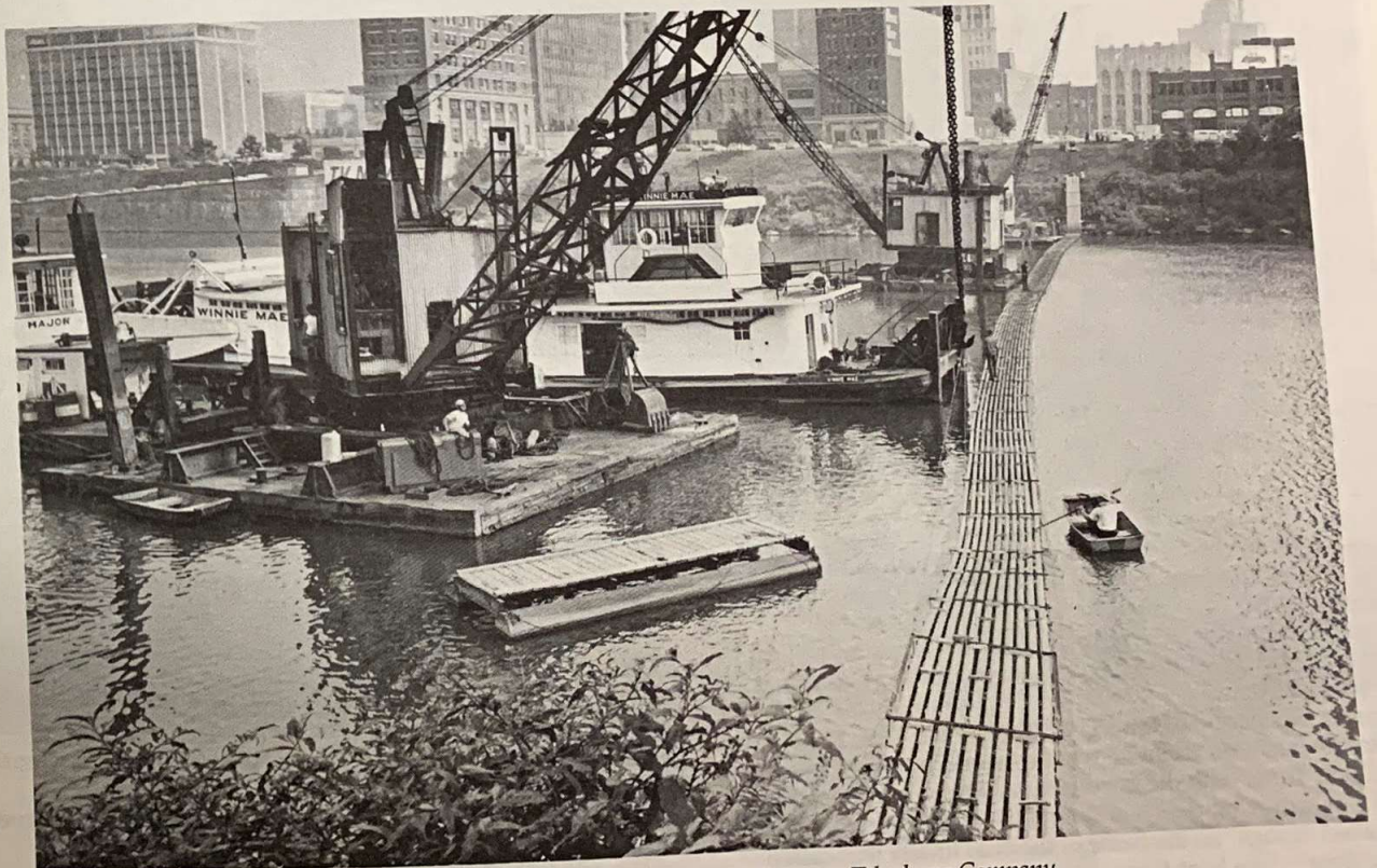
Laying cable for the Chesapeake and Potomac Telephone Company at Charleston, West Virginia
